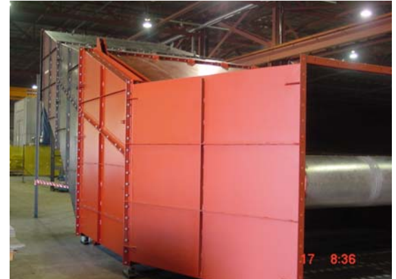
M&I's FD Fan Inlet Ducting for B&W, Coleson Cove, NB
