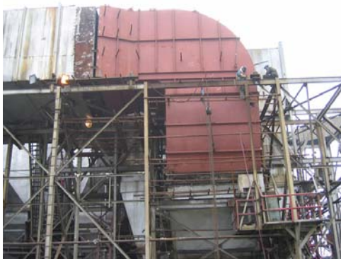
M&I's Installation for ID Fan Common Discharge Duct 210 MW Bandel Project, Unit # 5, WBPDCI, India
